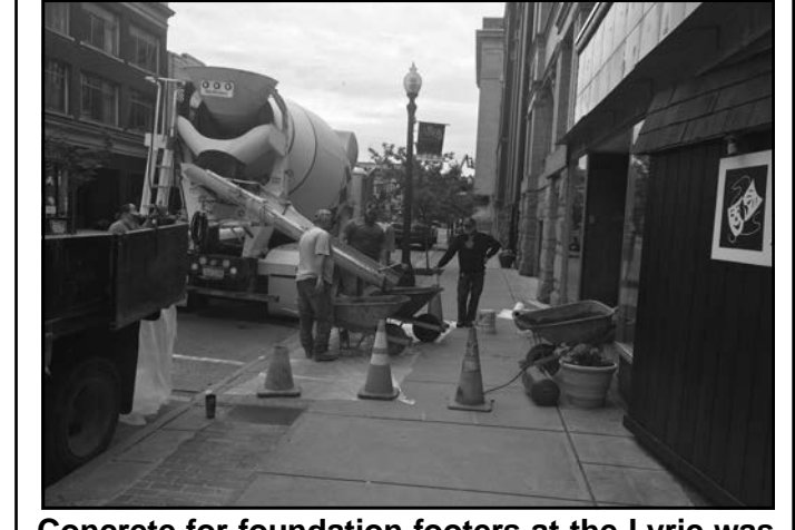
Concrete for foundation footers at the Lyric was taken to the job site via wheelbarrows.
